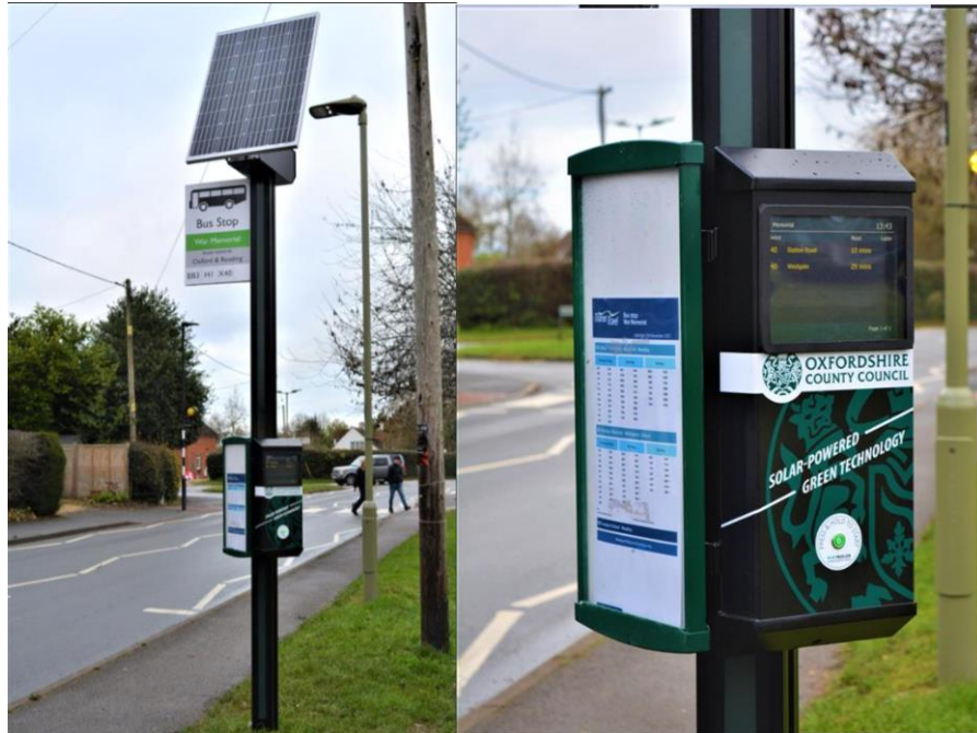
Figure 8 a pole mounted battery / solar 10" TFT display © M2M Tech
