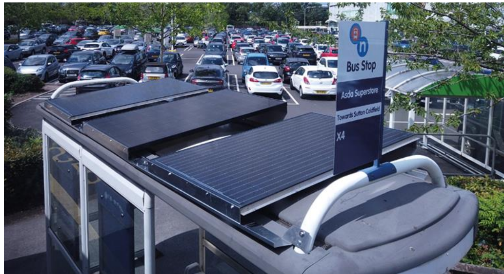
Figure 17 Shelter roof mounted solar panels in the West Midlands © Journeo
